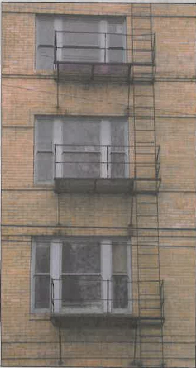
An old fire escape marks the Ferry Street side of the former St. Francis Hotel. The top three floors are vacant except for storage.
