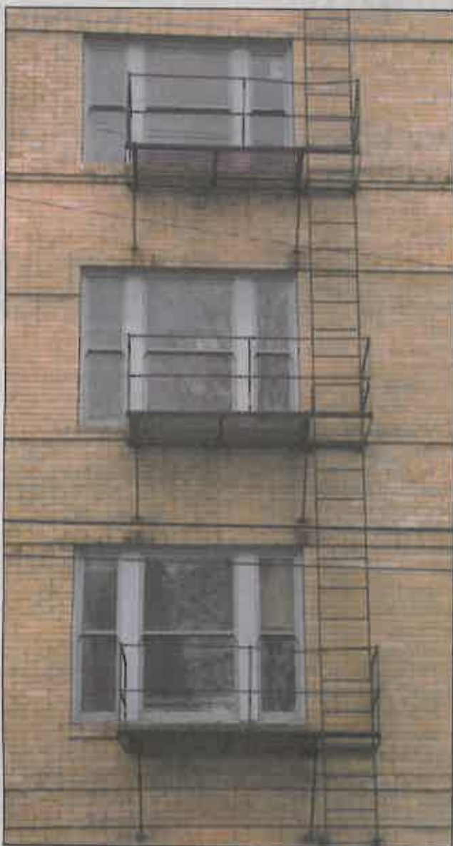
An old fire escape marks the Ferry Street side of the former St. Francis Hotel. The top three floors are vacant except for storage.
